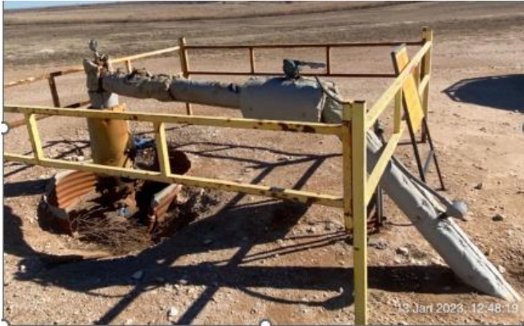
Tracing and Insulation – Wellhead
