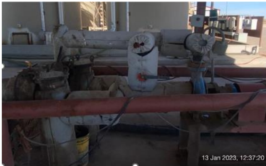
Tracing and Insulation pipes in unloading bay.
